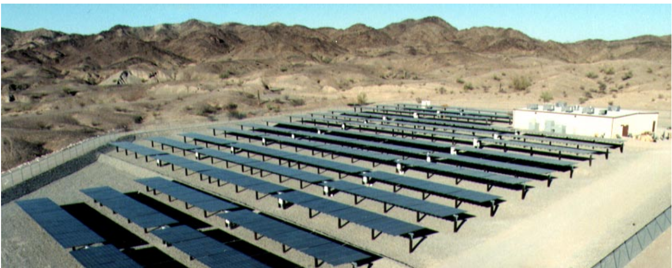
Fig. 1. The 450-kWp (DC side) photovoltaic array at Yuma Proving Ground in Arizona
