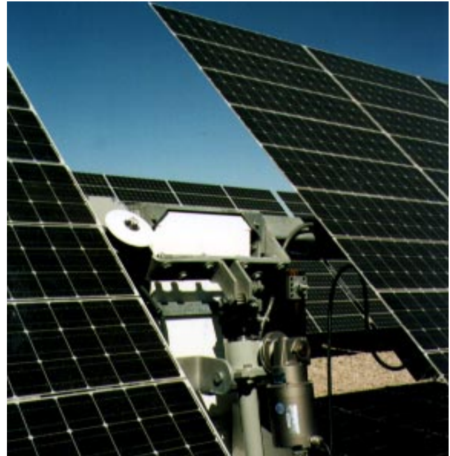
Fig. 4. Single-axis tracking system [4].
